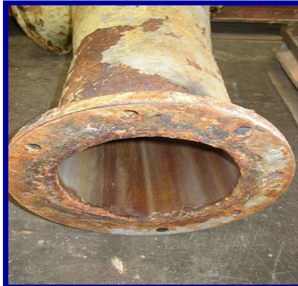
Severe undercutting & cavitation damage in the flange area.
