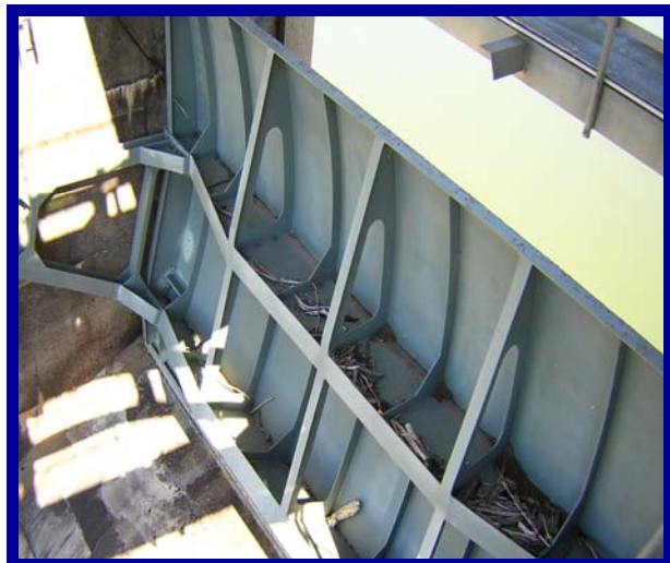
Visual inspection of one of the gates after service – showing no coating breakdown.
