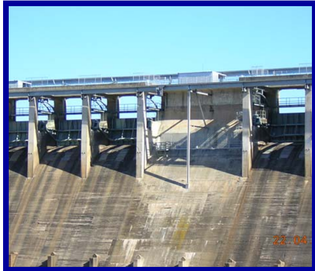
The spillway gates at Glenmaggie. Access to the gates was the first hurdle for Corrocoat.
